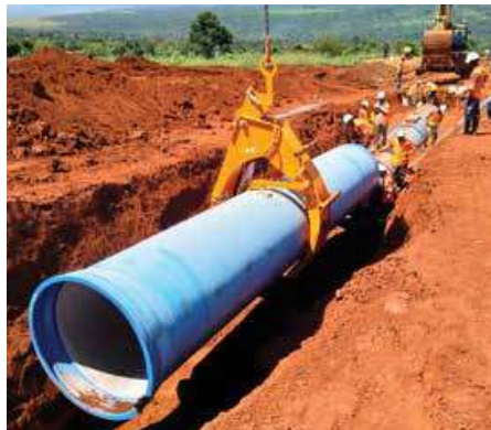
Preparation of detailed designs, tendering, and construction supervision of the Katosi-Kampala Transmission Mains (2016-2020)
