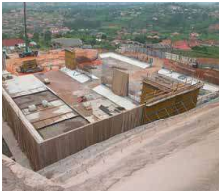
Design and construction supervision of a 15,000 m3 water tank at Ssonde under the Katosi Kampala Transmission Main Project
