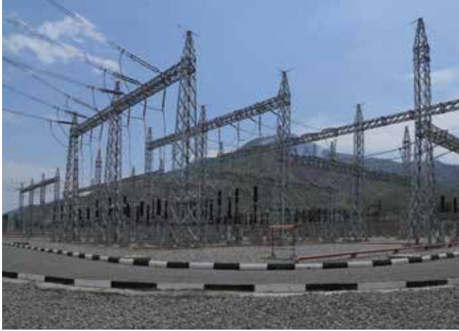
4 NKENDA Substation- Fort Portal
