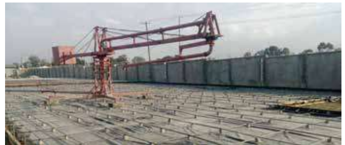
Figure 2: 14000 m 2 PT on ground, Vivo Energy Kenya Petroleum Depot, Nanyuki, Kenya
