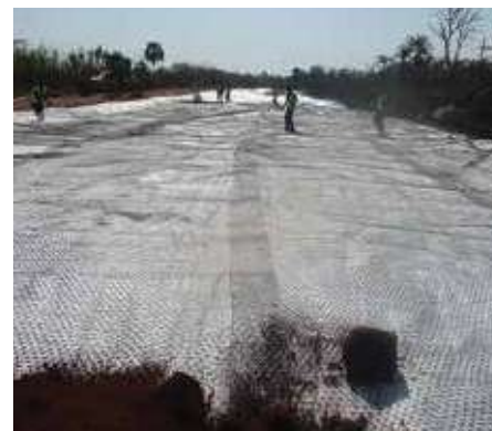
Design review and construction supervision of the upgrading of Kigumba – Bulima Road Project 2015– 2020 (placing of Geotextile earth reinforcing membrane)
