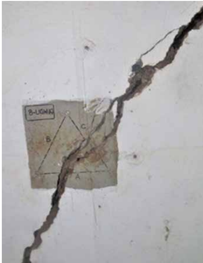
Figure 1: Crack at one of the turbine blocks in NPS
