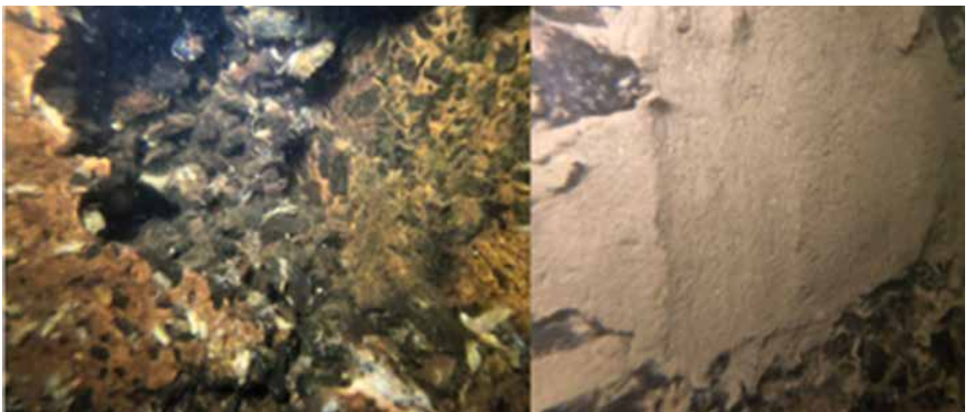
Figure 3: Before and after images of specialized underwater diver remedial repairs at Nalubaale in 2019
